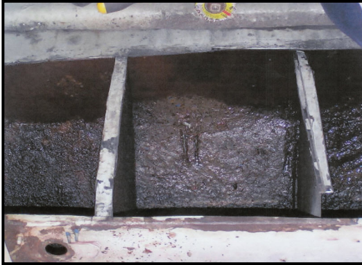
Tank, with front removed, showing baffles and sludge!
