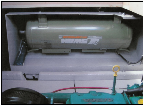
New tank showing filler at left and fuel outlet below
